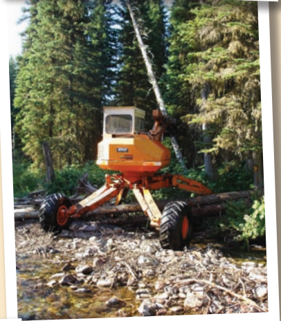
A helicopter and spider excavator were used to build large wood structures designed to provide bull trout habitat, trap spawning gravels, and increase channel complexity
