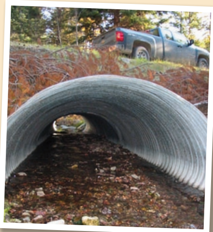
"Fish-Friendly" culverts are being installed at road crossings on Plum Creek land throughout Montana
